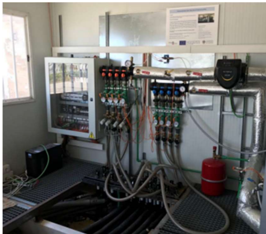
Figure 8: Connection of pipes from new BHEs to the control unit inside the UPV laboratory.
