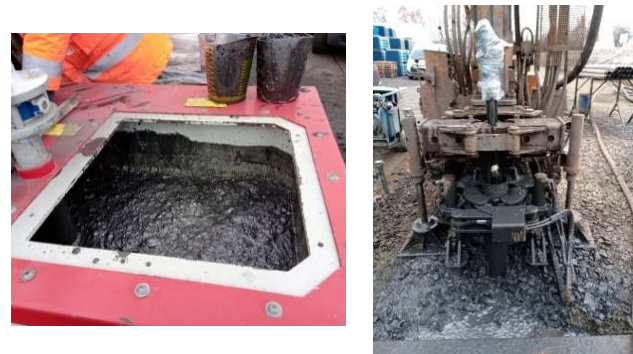
Figure 12: GEOCOND grout in the colloidal mixer (left) and exiting the borehole top (right).
