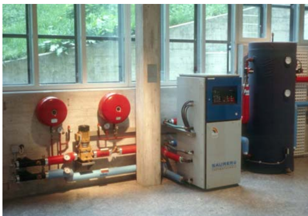
Figure 17: GSHP in the museum of natural history in St. Gallen, Switzerland (photo from 1993)
