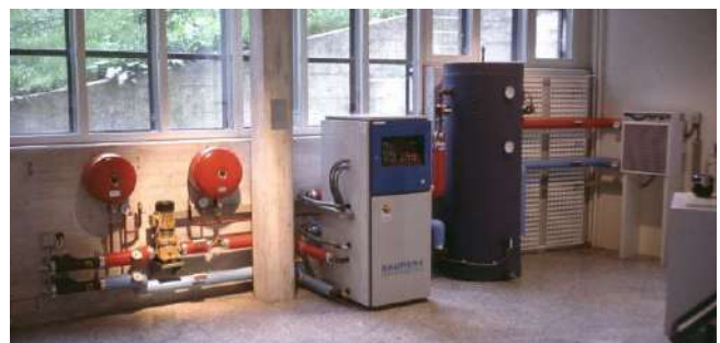
Figure 34: GSHP in the museum of natural history in St. Gallen, Switzerland (photo from 1993); connection to BHE to the left, and the fan-coil unit in the far right.
