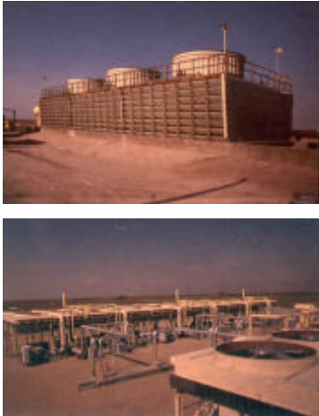
Fig. 6: Wet cooling tower (above) and dry coolers (below) for geothermal power plants [4]
