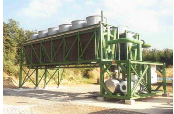
Fig. 8: ORC unit in Bad Blumau, Austria (250 kW el. Output): Evaporator, turbine, condenser and controls in the frame to the lower right, air coolers for re-cooling the condenser in two parallel racks to the upper left (cf. fig. 7) (Photo ORMAT, Israel)
