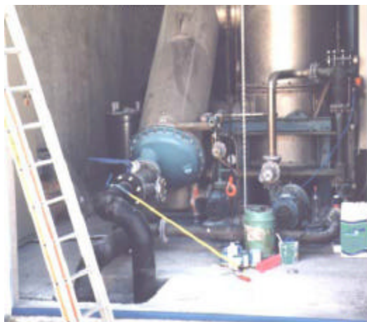
Fig. 13: The geothermal desalination unit for Kimolos island (photo: CRES)
