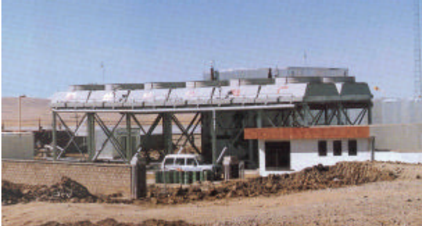
Fig. 9: Frame with evaporator, turbine, and condenser of ORC-plant in Wabuska, Nevada, USA (above) and complete view with air coolers of plant in Nagqu, Tibet, China (below) [4]
