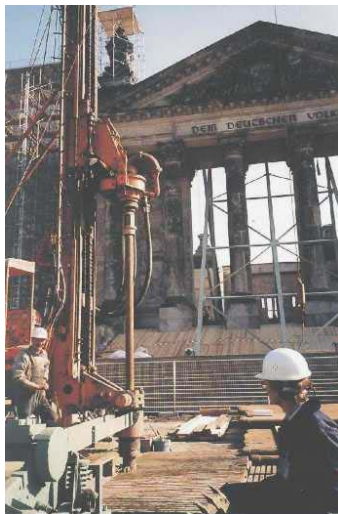
Figure 3: Drilling of the first deep well in front of the main entrance in 1996, while the complete interior of the building has been removed before rebuilding (photo: GTN)
