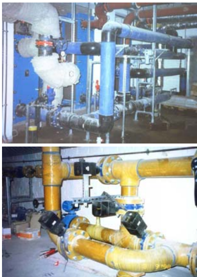
Figure 6: Groundwater-bearing pipe connections at the entrance into the Reichstag building, cold storage system (above) with heat exchangers to the left, and heat storage system (below) (photos: GTN)
